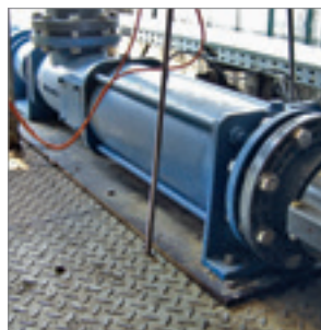
Pumping substrate between fermenters
